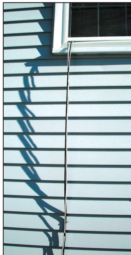
The direct-bury coax makes a discreet jaunt into the bedroom window.
